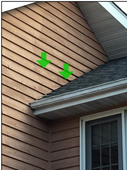
Cracked, split or broken
