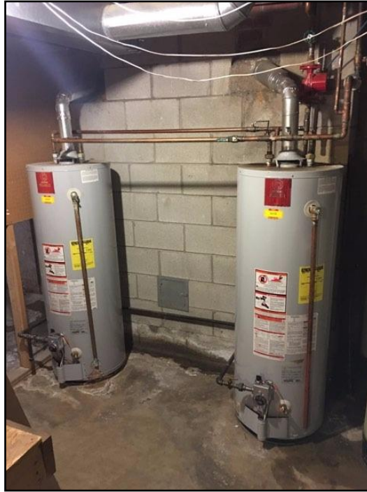
The estimated age of the water heater...
