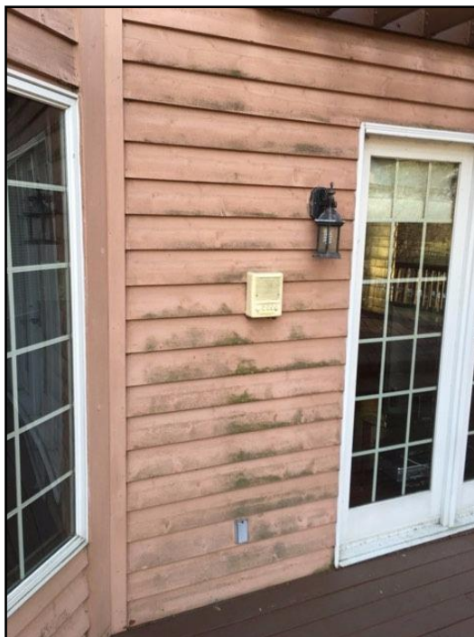
Paint or stain - needed
