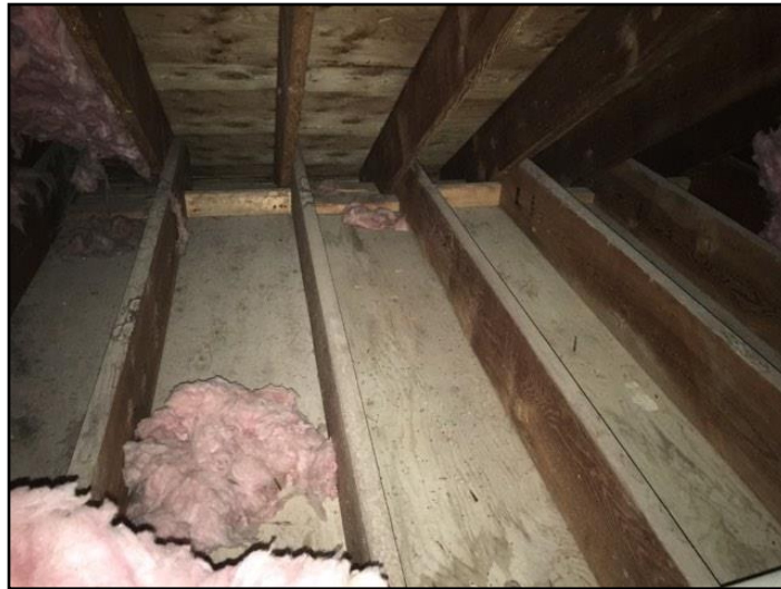
Gaps or voids
