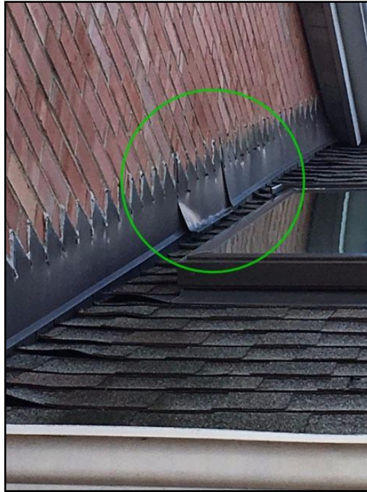
Loose sidewall flashing
