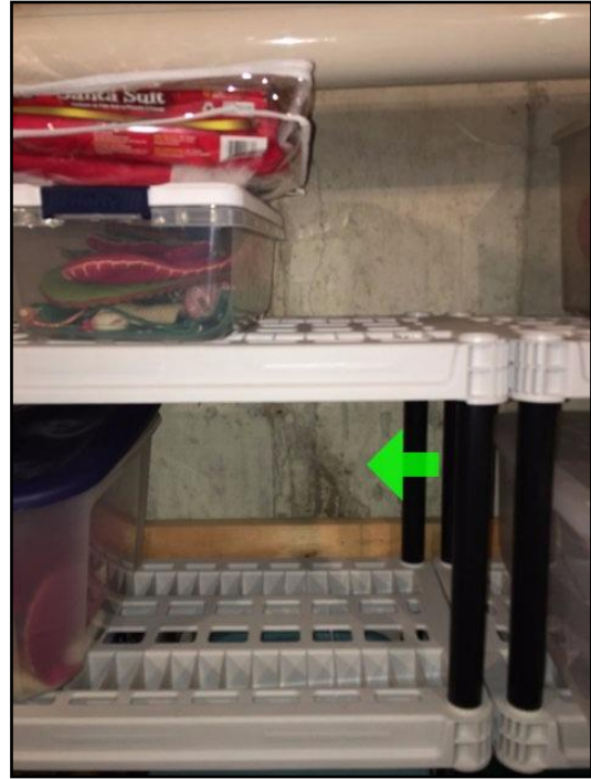
Cracked with signs of seepage
