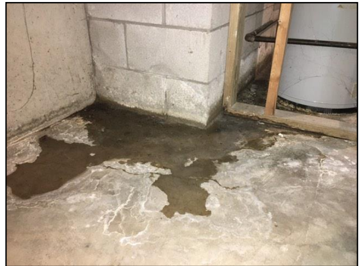
Dampness on floor or walls
