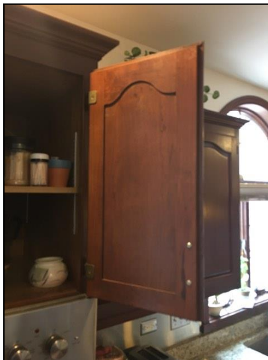
Doors or drawers missing or loose
