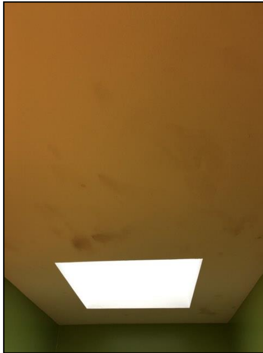
Inadequate air movement
