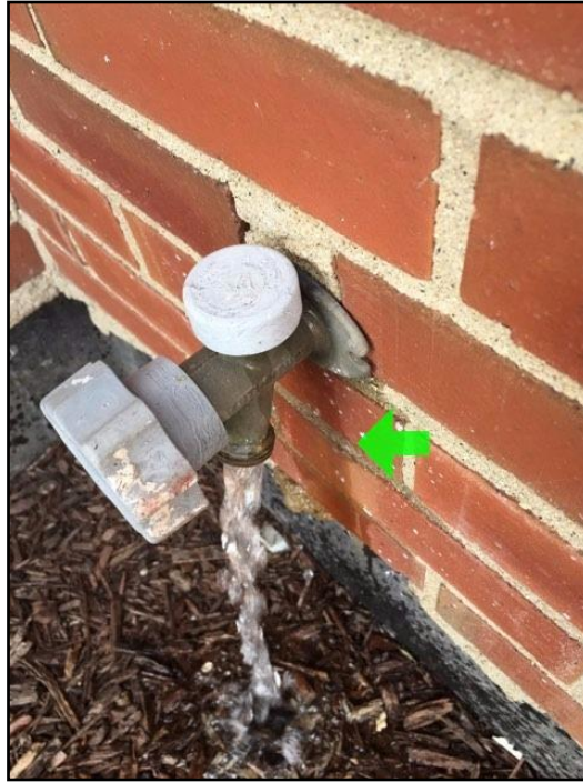
Leak or drip
