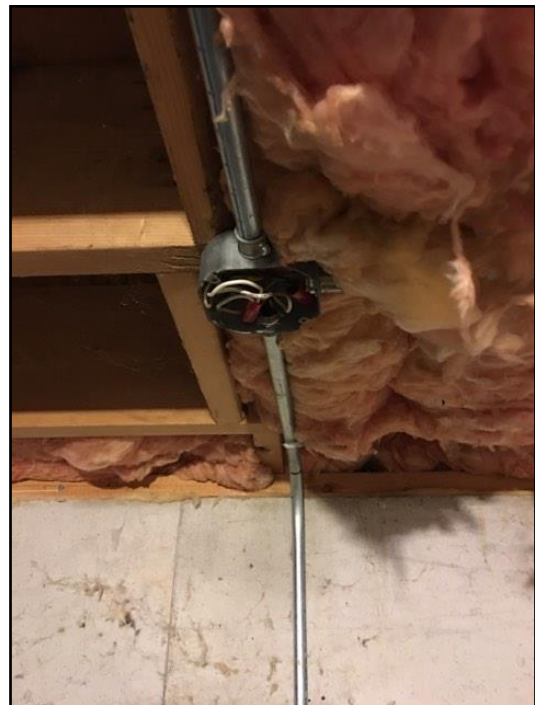
Cover loose or missing
