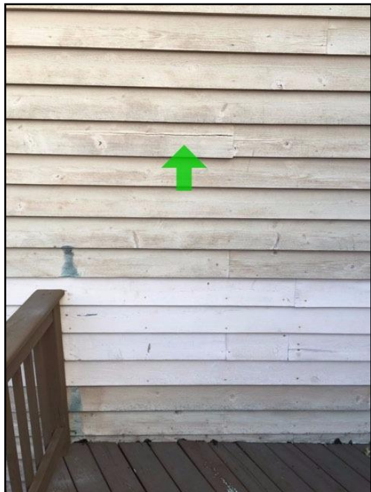
Cracked, split or broken
