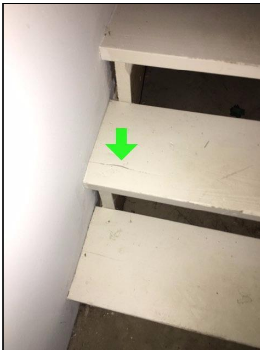
Worn or damaged
