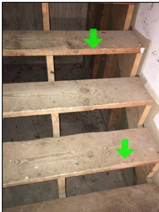
Worn or damaged
