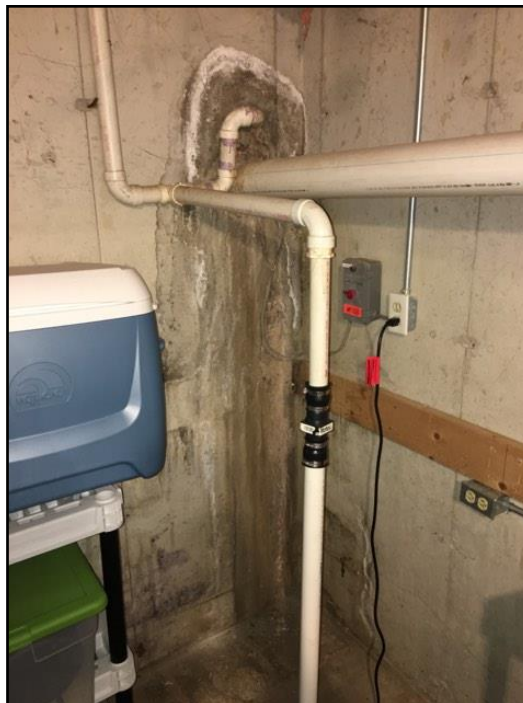
Cracked with signs of seepage
