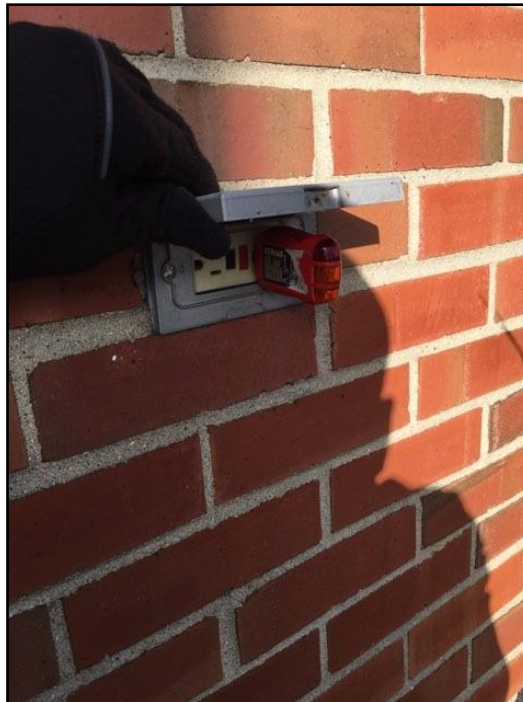
Test faulty on Ground Fault Circuit...
