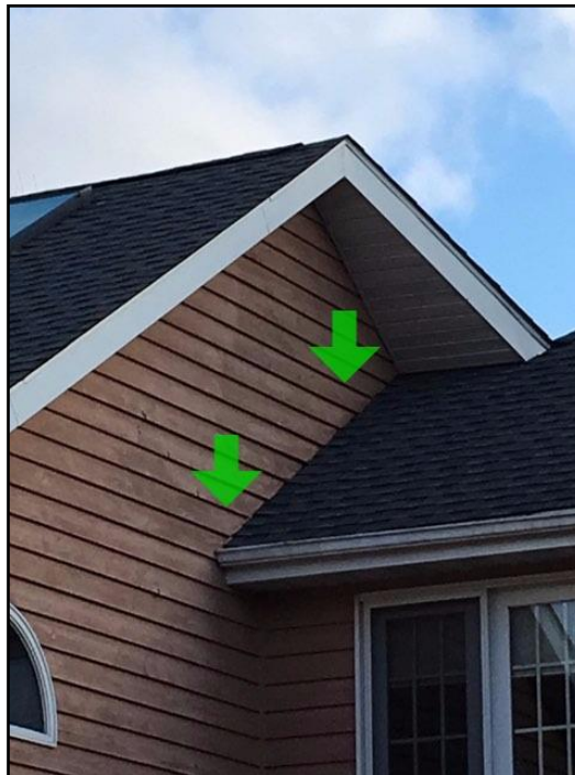
Siding not cut back from roof
