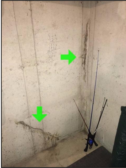
Cracks with signs of seepage
