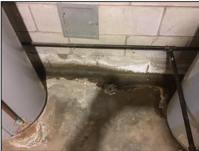
Dampness on floor or walls
